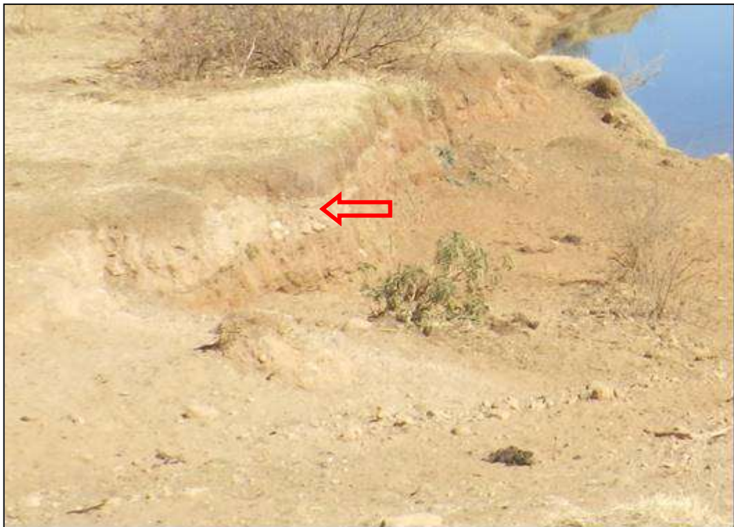
Photo 16. Same as above, close up view of the suspended gravel layer (arrow).
